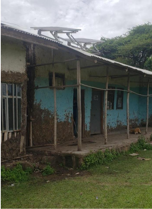
Figure 12: Health post at Dodota chire Kebele use solar as source of energy
